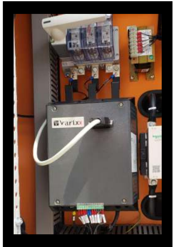
Cable Connection Example
