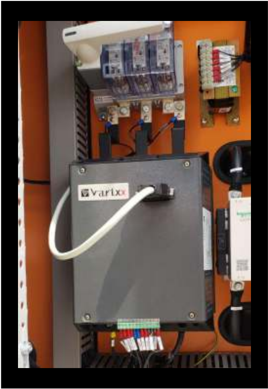
Cable Connection Example
